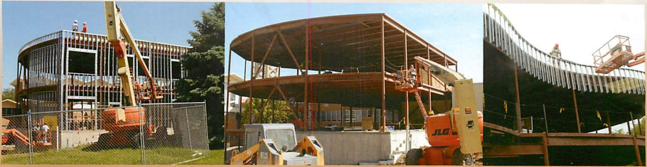
Scheduled construction continues on the new Education Wing building on the Logan campus. The building is expected to be completed in January 2012.
